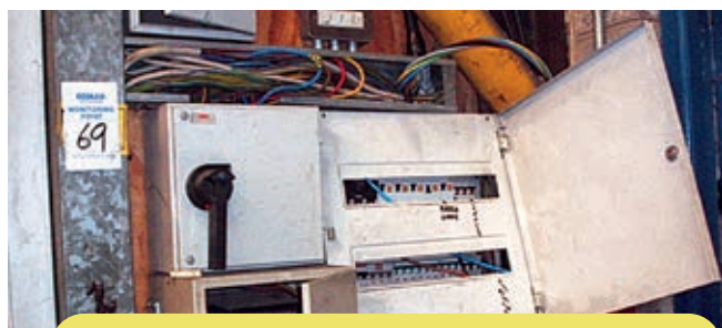
Fig 7.4 Installations like these can lead to inadvertent contact and electrocution
