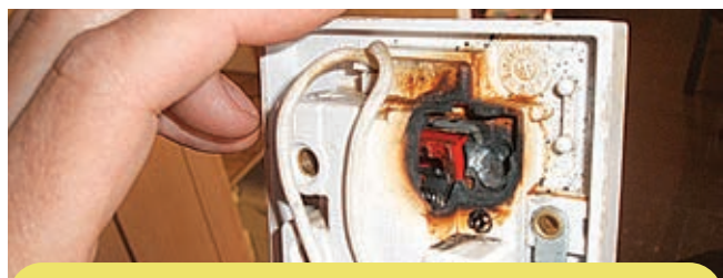
Fig 7.3 Potential ignition source from electrical equipment
